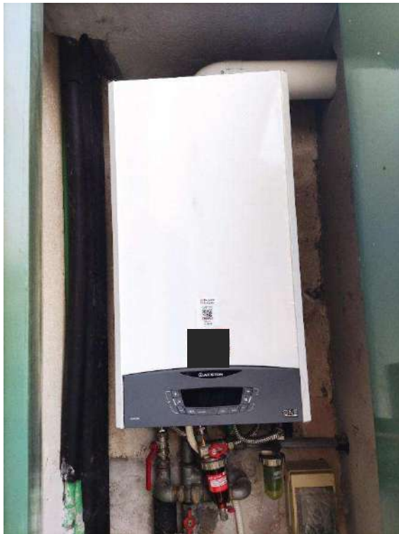
CALDAIA A GAS
