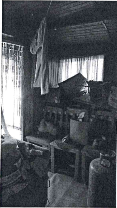
SUB 3 - VERANDA ABUSIVA
