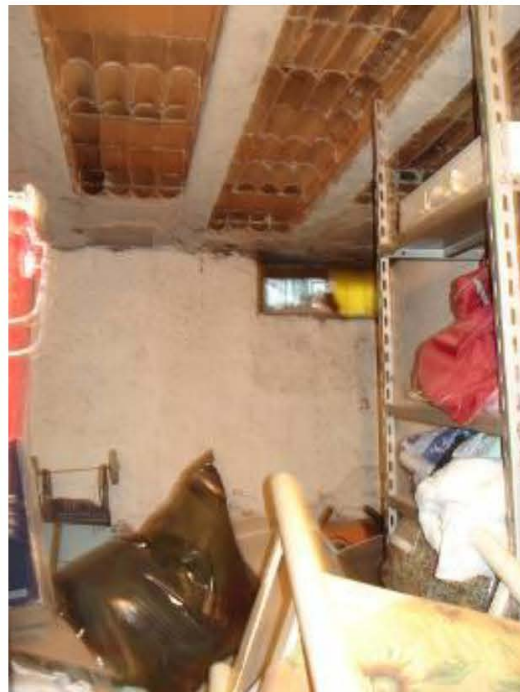
locale piano S-1
