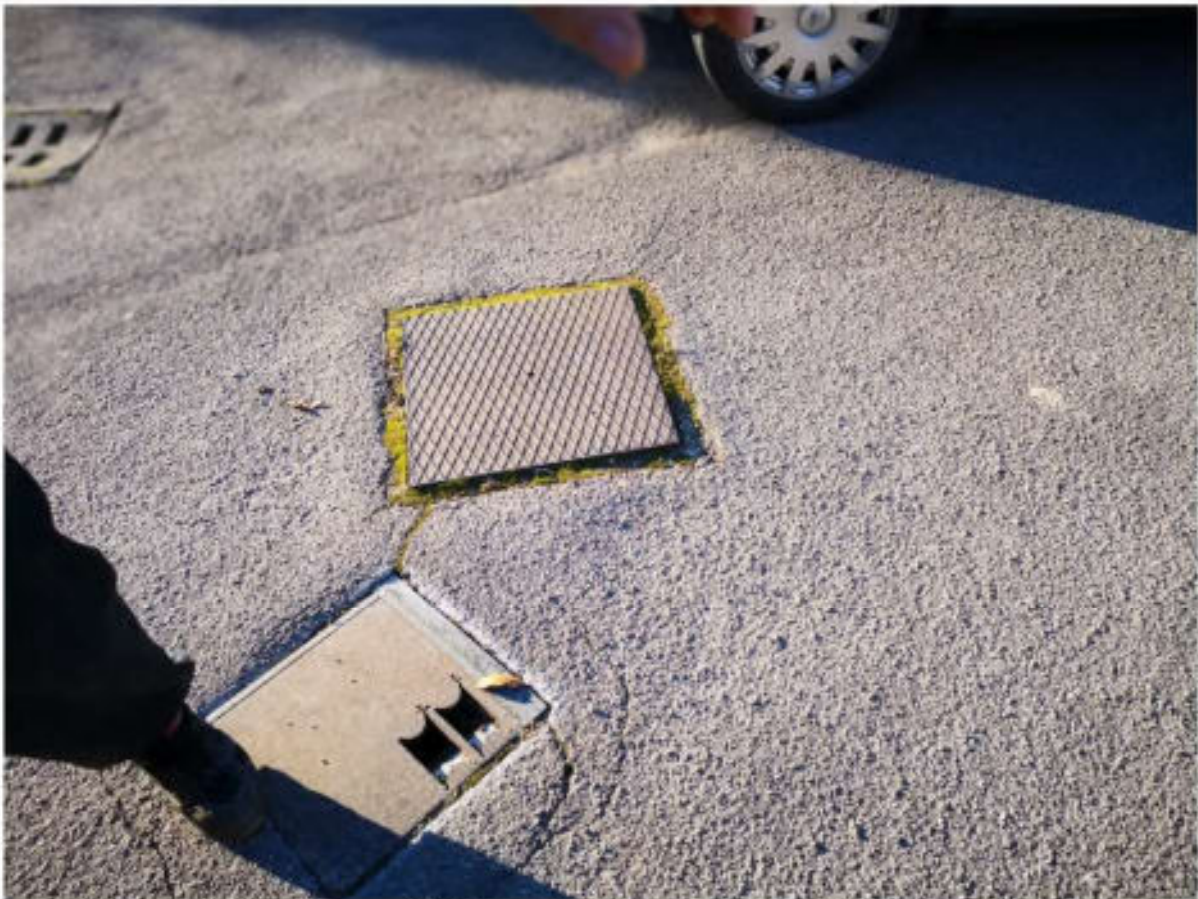
1.69 pozzetti cisterna gasolio
